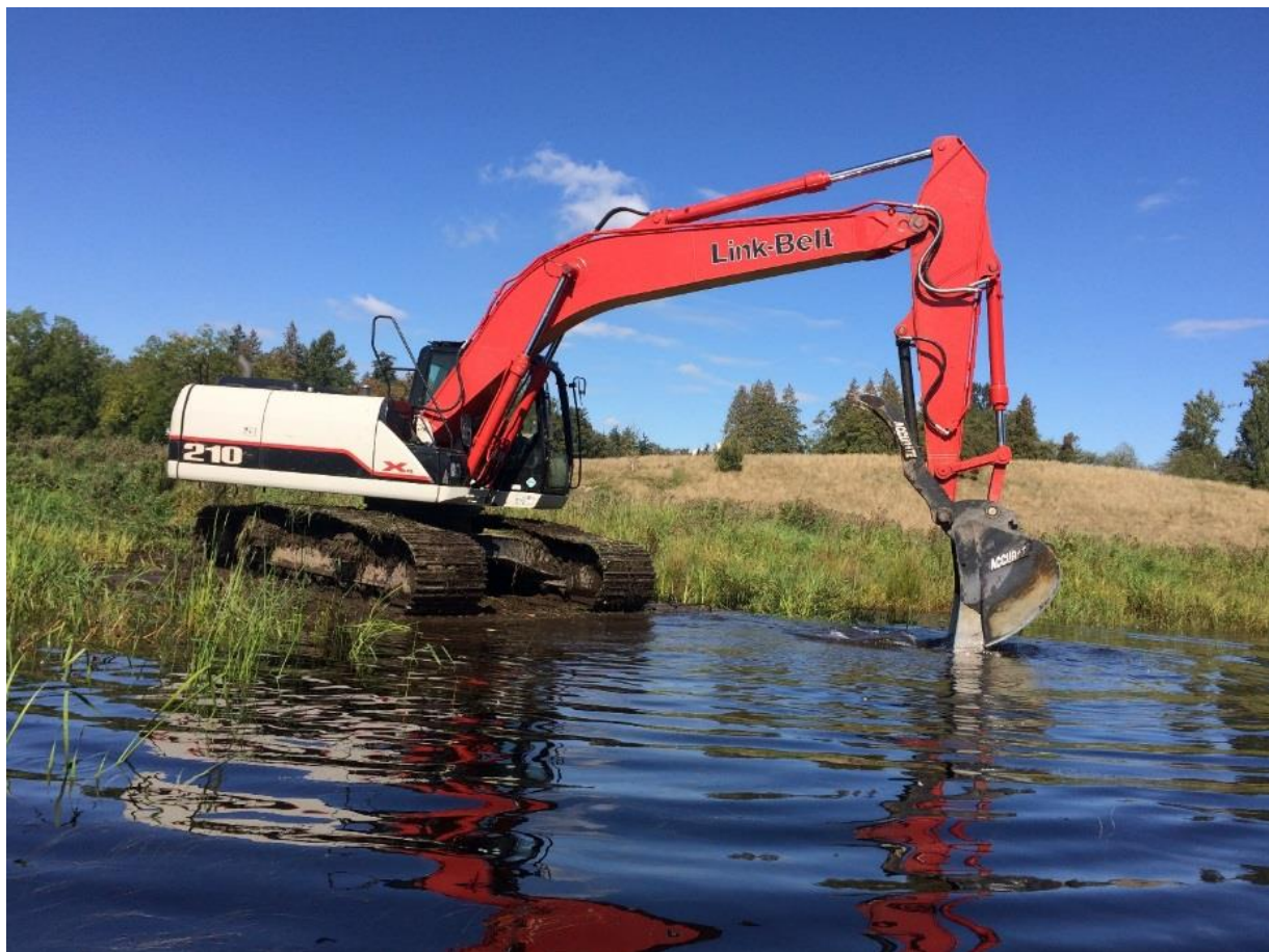
Figure 4: The majority of construction works were completed from swamp pads, while digging in the water.
